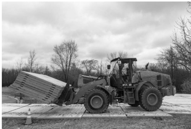
FIGURE 1.3 CLT mats used as temporary roads for construction purposes. (Courtesy of Sterling Lumber.)
